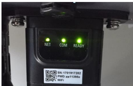
Figure 74 - Final status of LEDs
