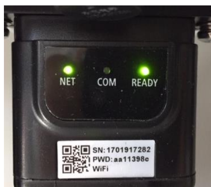
Figure 75 - Irregular communication status between inverter and adapter
