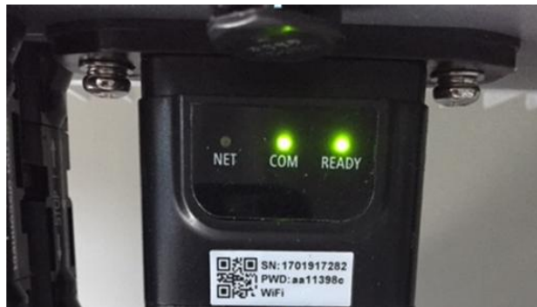
Figure 69 - Initial status of LEDs
