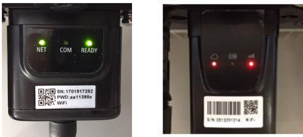
Figure 54 - Irregular communication status between inverter and Wi-Fi
