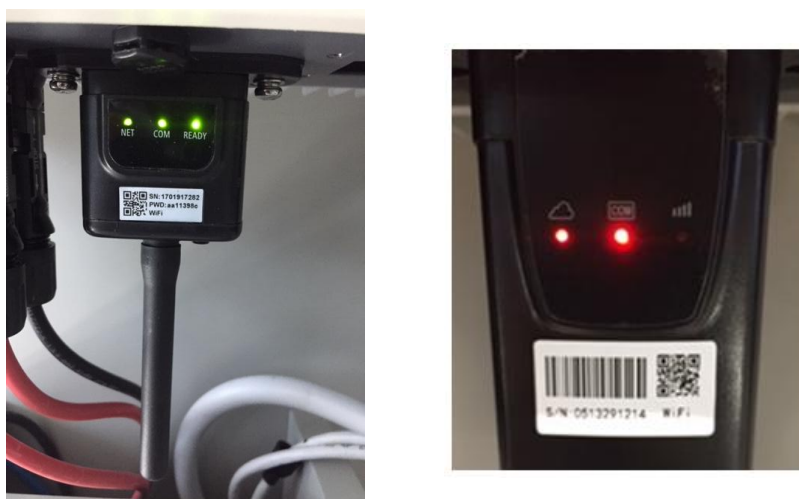
Figure 52 - Final status of LEDs
