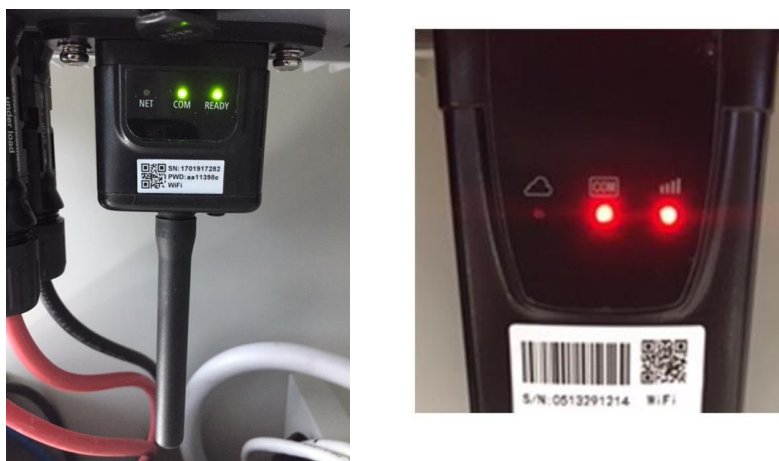
Figure 51 - Initial status of LEDs
