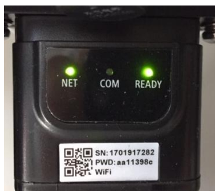
Figure 71 - Irregular communication status between inverter and adapter
