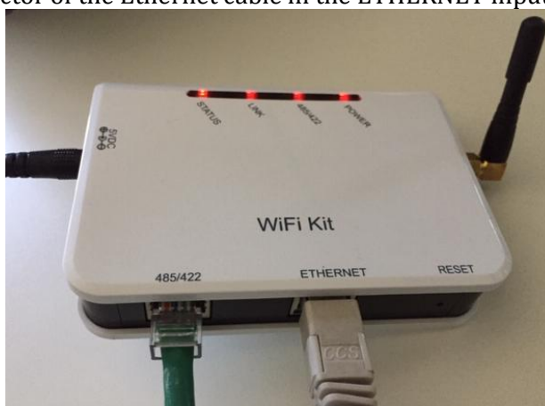
Figure 81 – Ethernet cable connected to the datalogger
